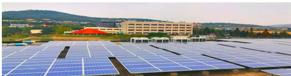
Solar panels on the roof of Qingdao DIC Finechemicals
