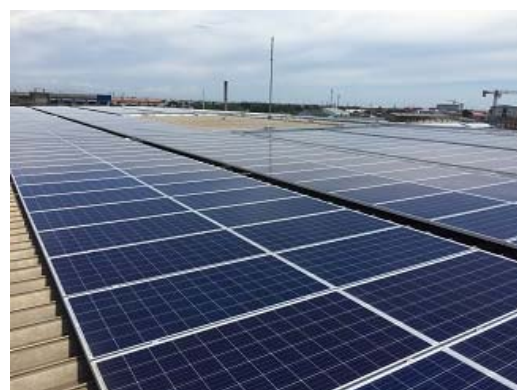
Rooftop solar panels
